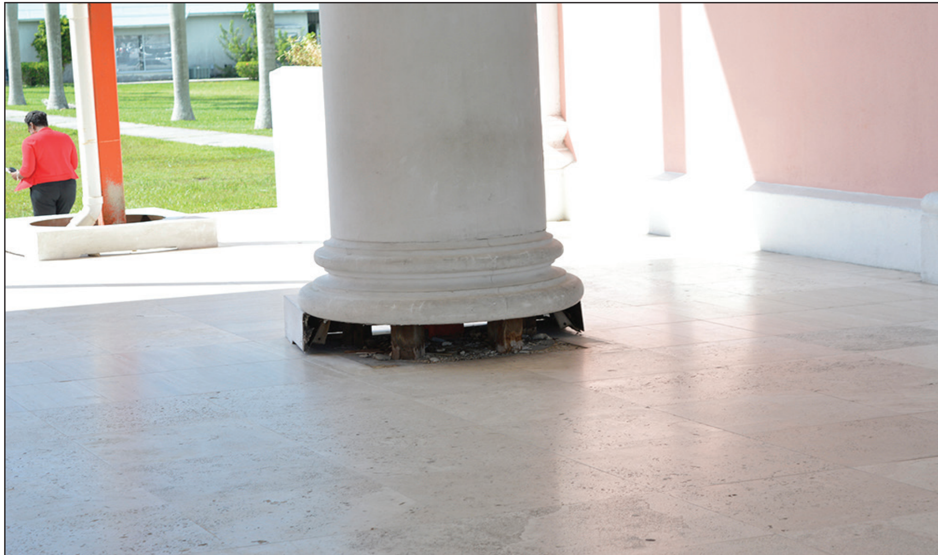
BAD CONDITION – Local attorneys continue to voice concerns over the state of the Garnet Levarity Justice Center.
