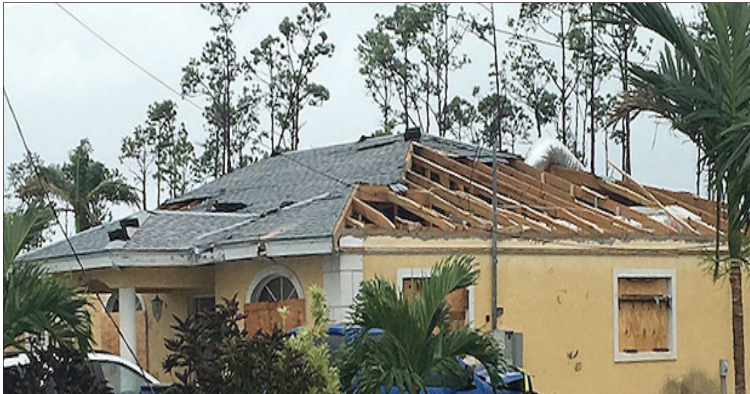
TORNADO DAMAGE – Several homes in the Imperial Park Subdivision and businesses in the area sustained minimal to extensive damage yesterday as a tornado ripped through portions of Grand Bahama.
